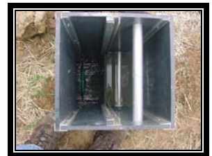
Close up of water Control Structure
