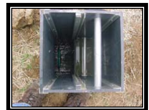
Close up of water Control Structure
